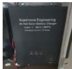
Plate 26. Solar Battery charger
