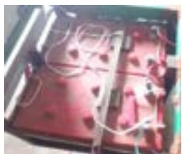
Plate 25. Battery/power Storage of the carrier
